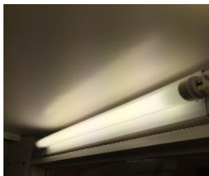
Figure 1: Existing Bare Fluorescent Lamp Mounted in Top of Display Cases
